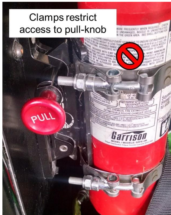
Figure B-47: Incorrect orientation of extinguisher clamps.
